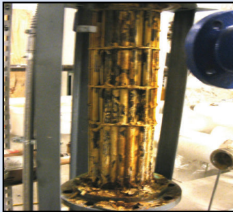
Limescale buildup on the heat exchanger before Flow-Tech
