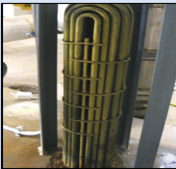
Flow-Tech removed and prevented new scale from forming and restored heat exchanger performance
